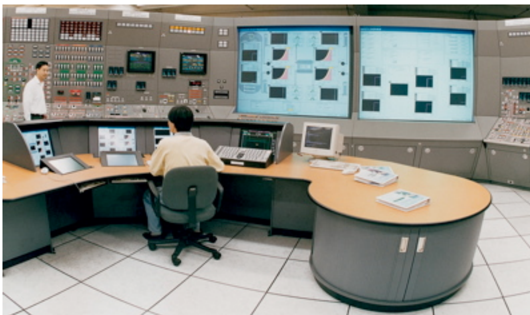
Figure 1 - Qinshan Control Room and Central Panel Wall Displays.
